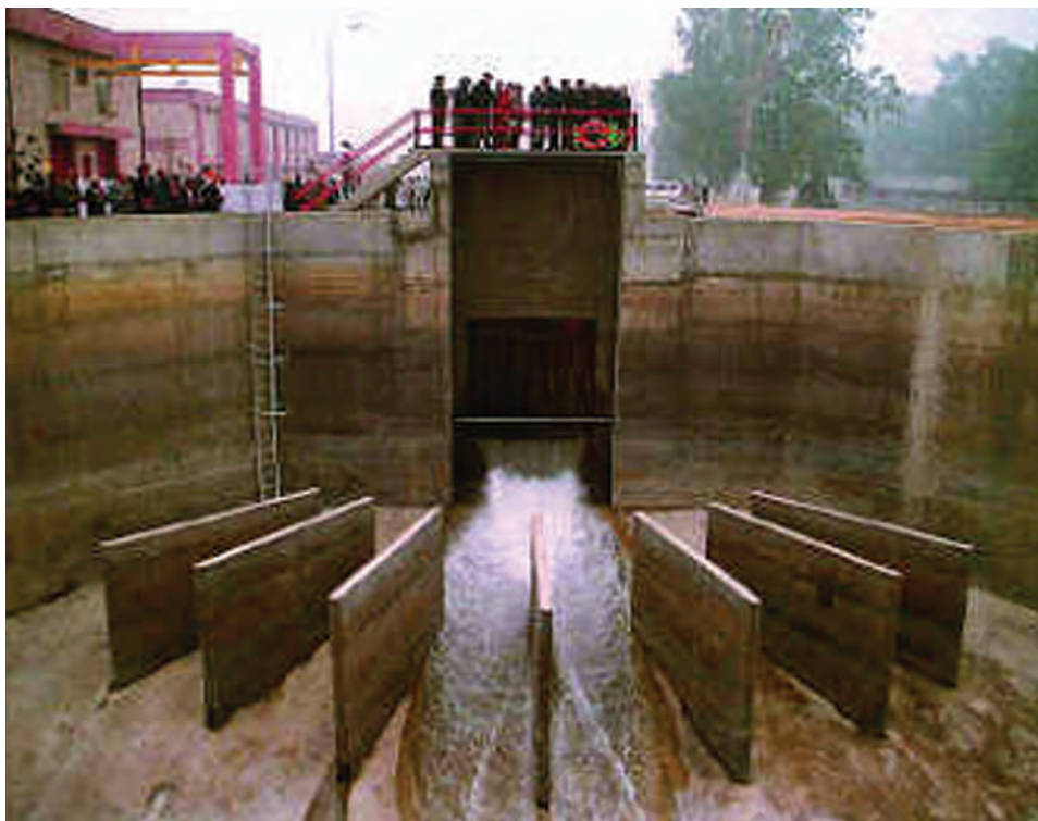
Fig. 18.10 : Water treatment plant
